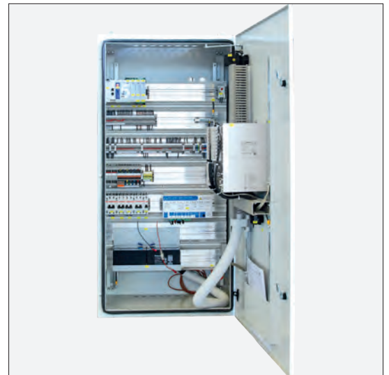
QU protective cabinet with SEG Woodward MRA4
